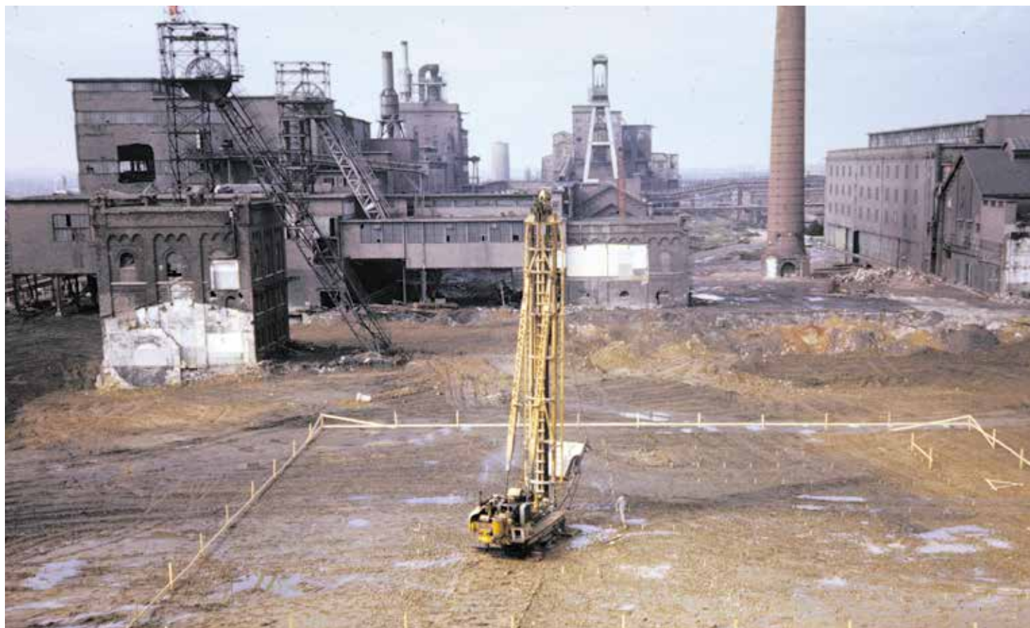
Start of the construction of the Heerlen office of Statistics Netherlands on the site where part of the Oranje-Nassau I coal mine once was. Photo: J.H.M. Wismans - Historisch Centrum Limburg
